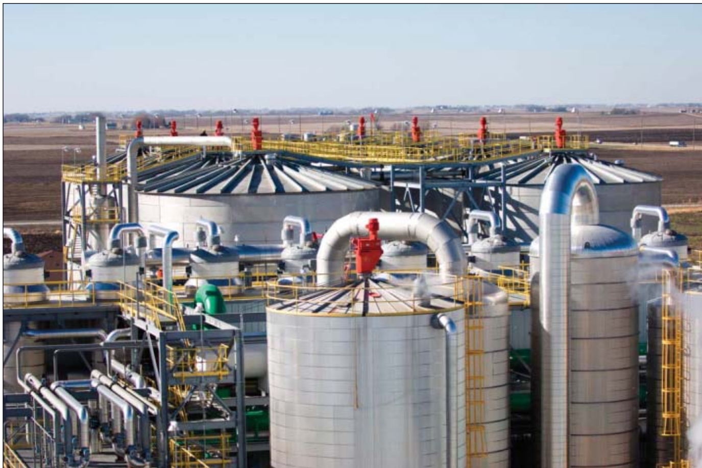
VeraSun Energy Corp., Brookings, SD, started up this ethanol plant, one of the largest in the US, outside Fort Dodge, Iowa, in October 2005. The plant can convert 39 million bushels/year of corn into 110 million gal/year of ethanol. Photo from VeraSun.
